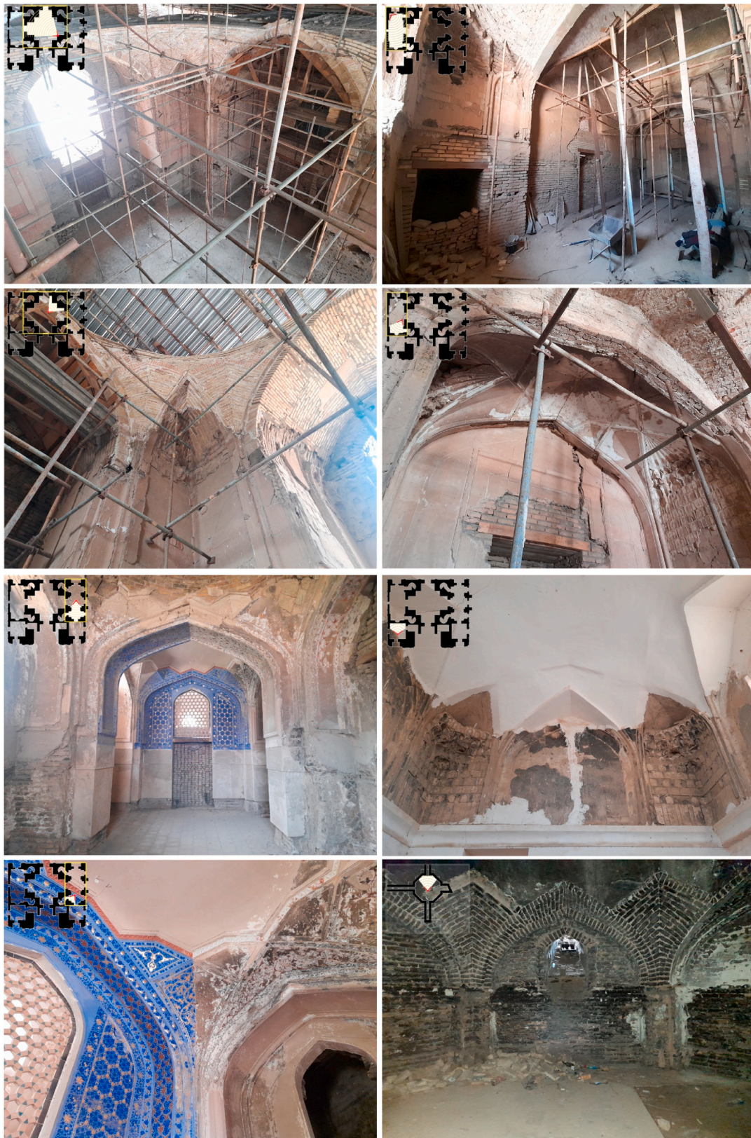
Fig. 2. Current status of the interior domes: (a–b) Ruins of the central hall (Space 1a); (c) The reconstructed segmental dome of the masjid (Space 6a); (d) Original ribbed vaulting above the mihrab; (e–f) The preserved dome in the southern hall and its details (Space 3); (g) The basement (Space 0) showing saline damage.
